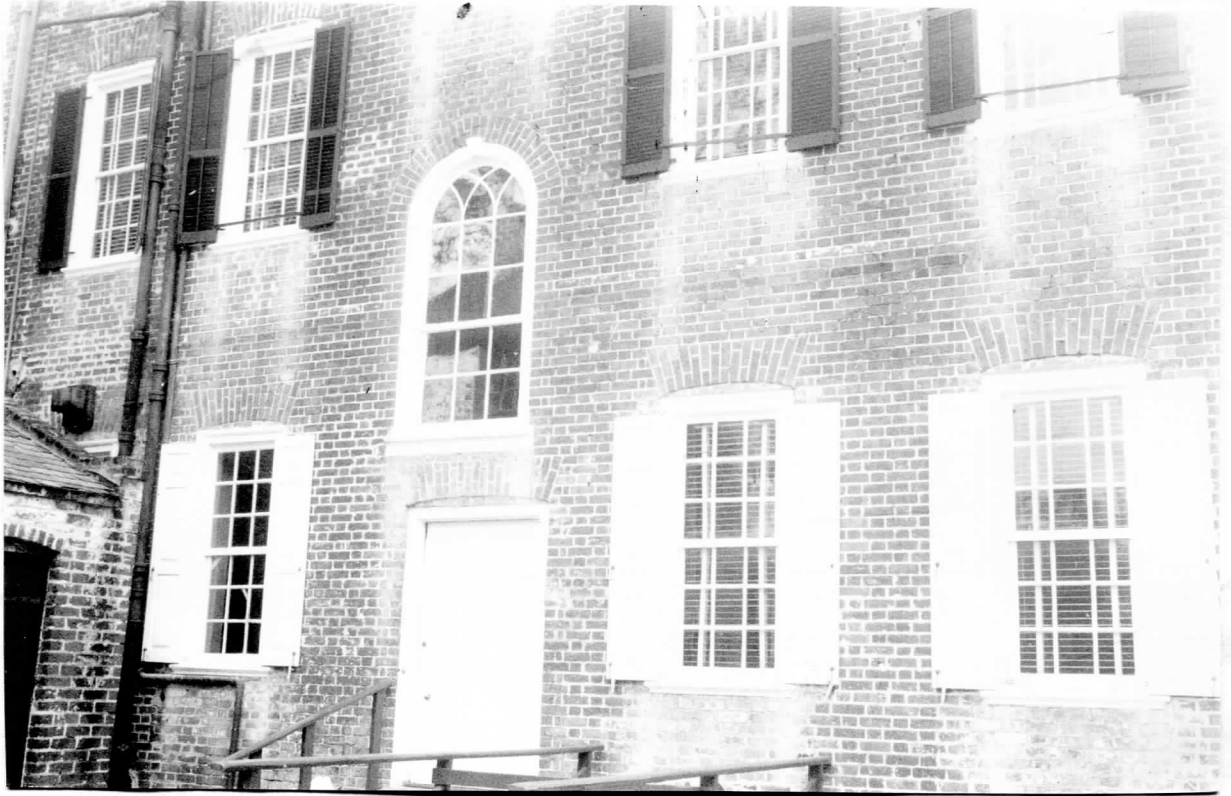
Figure 18. Photograph of the back of the Heyward-Washington house showing the line of brick across the palladian window which does not correspond to the Flemish bond pattern of the rest of the wall.
